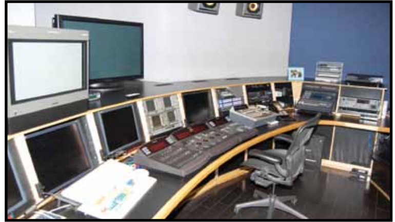
View of (4) Telecine Suites
