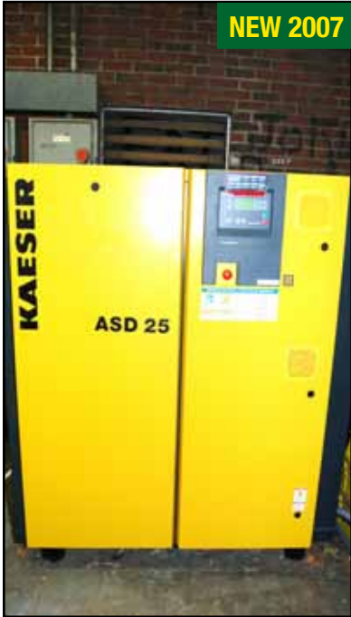
KAESER AIR COMPRESSOR
